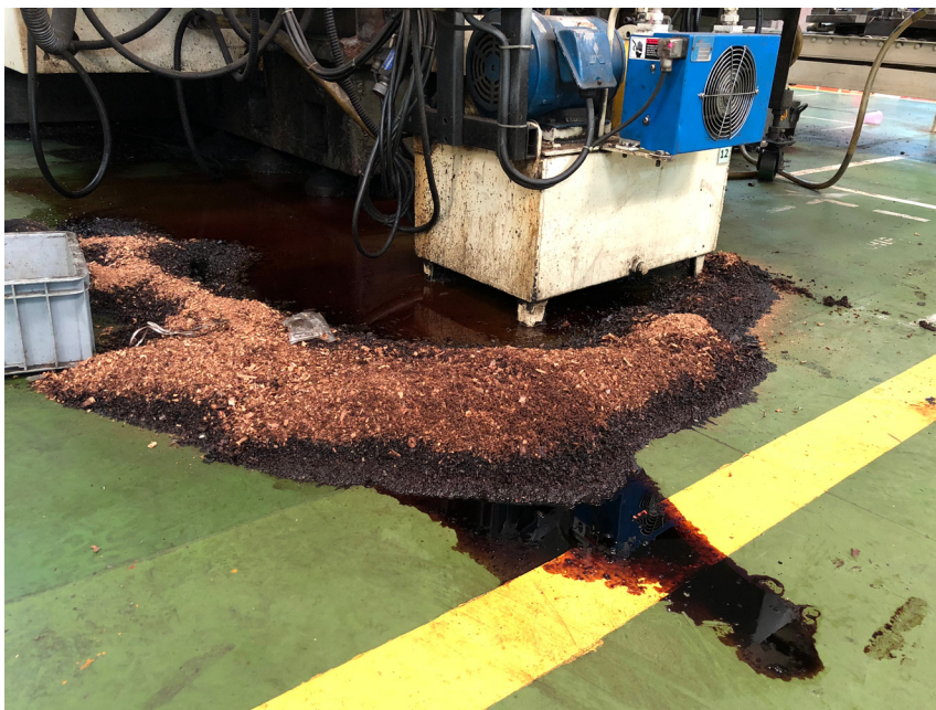
Hydraulic systems use various types of fluid that can be messy, slippery and hazardous to humans and the environment. As hydraulic fluids lose effectiveness over time, special care and regular maintenance is critical.
